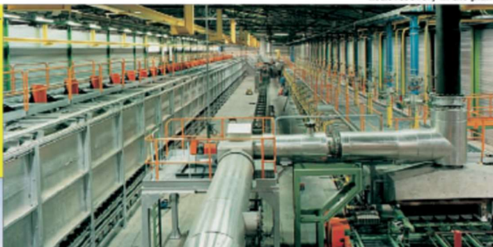
High priority is given to heat recovery in the plant.
