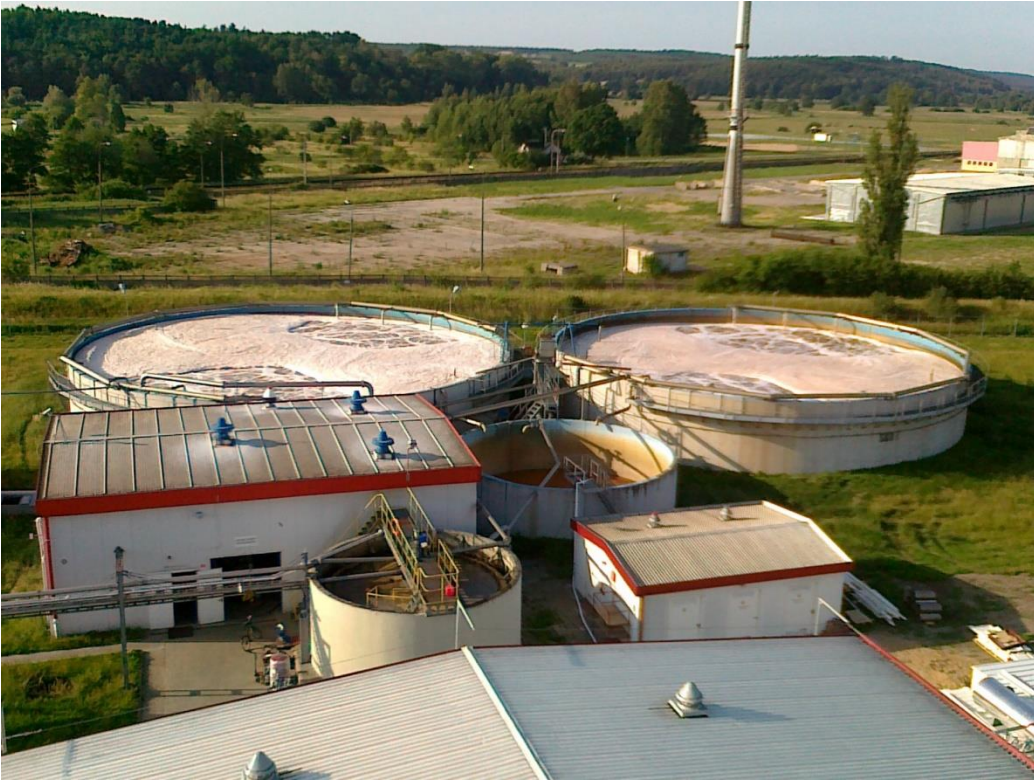
Figure 18 Aerobic stage - SBR's
