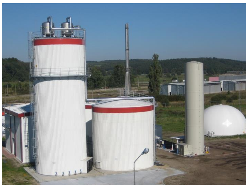
Figure 13 Shown from the left: anaerobic reactor, acidification tank, desulphurization column and storage tank (FFP SA).
