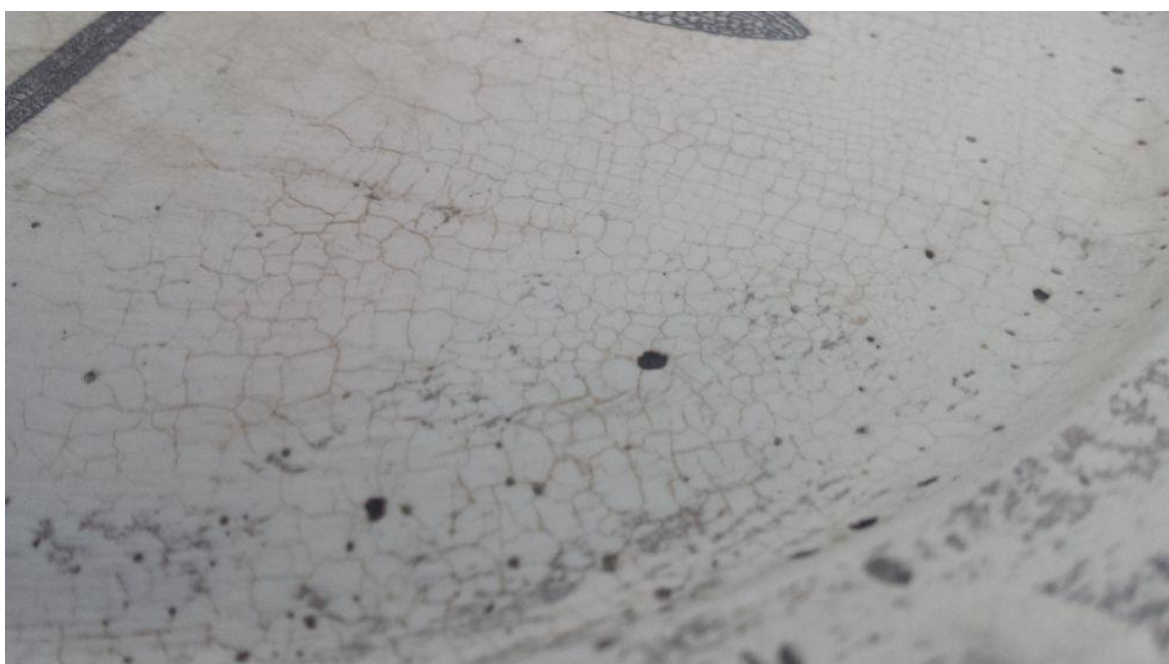
Figur 8. Krackelerad betong. (Eva-Marie, 2015)
