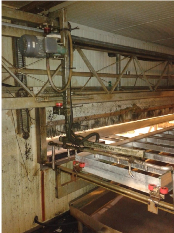
FIGURE 9. Inside mechanism of the washing machine (Fedotova 22.10.2015)
