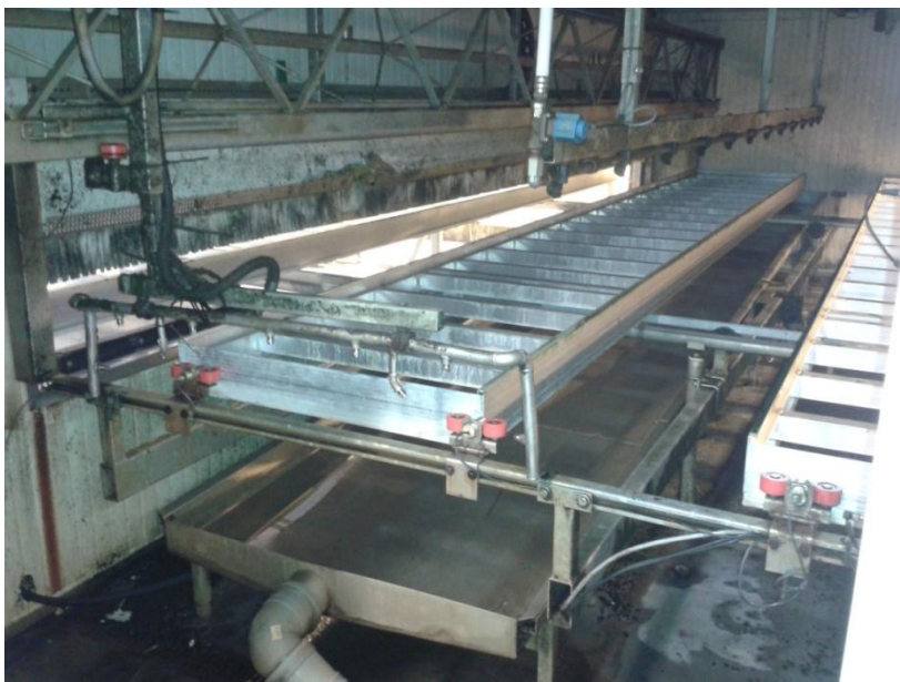
FIGURE 1. Inside mechanism of the washing machine (Fedotova 22.10.2015)
