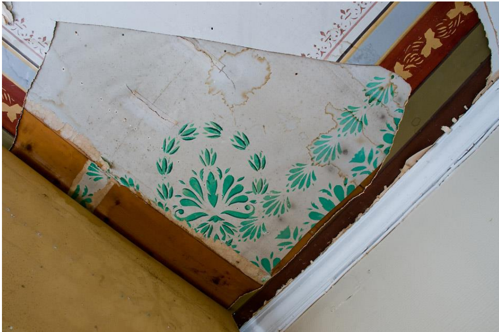
Picture 12. A beautiful decorative painting was discovered during the renovation of Hovila manor (Päärakennuksen restaurointi).
