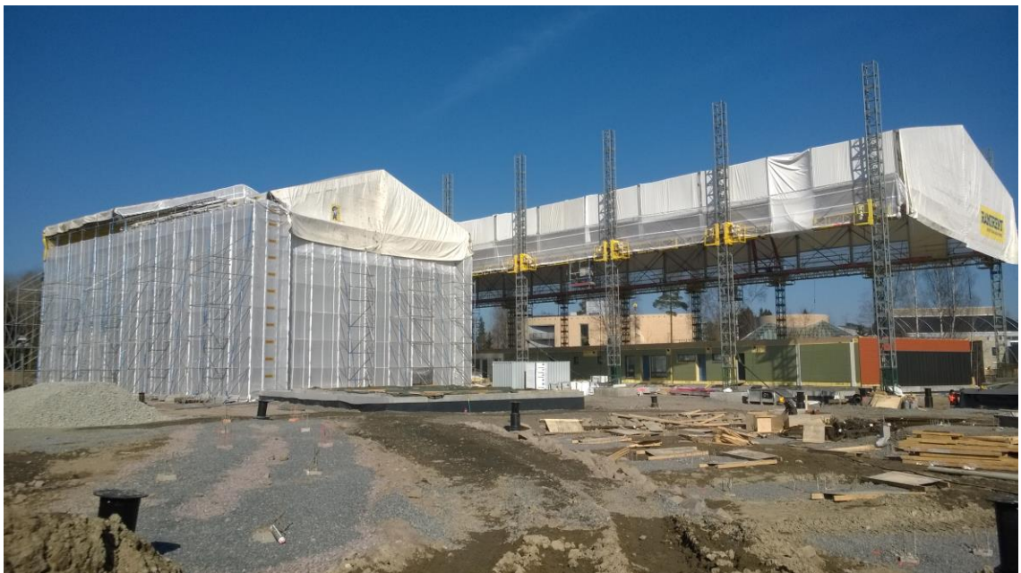
Figure 1. The two systems assembled. Layher on the left, Gibson Tower on the right.
