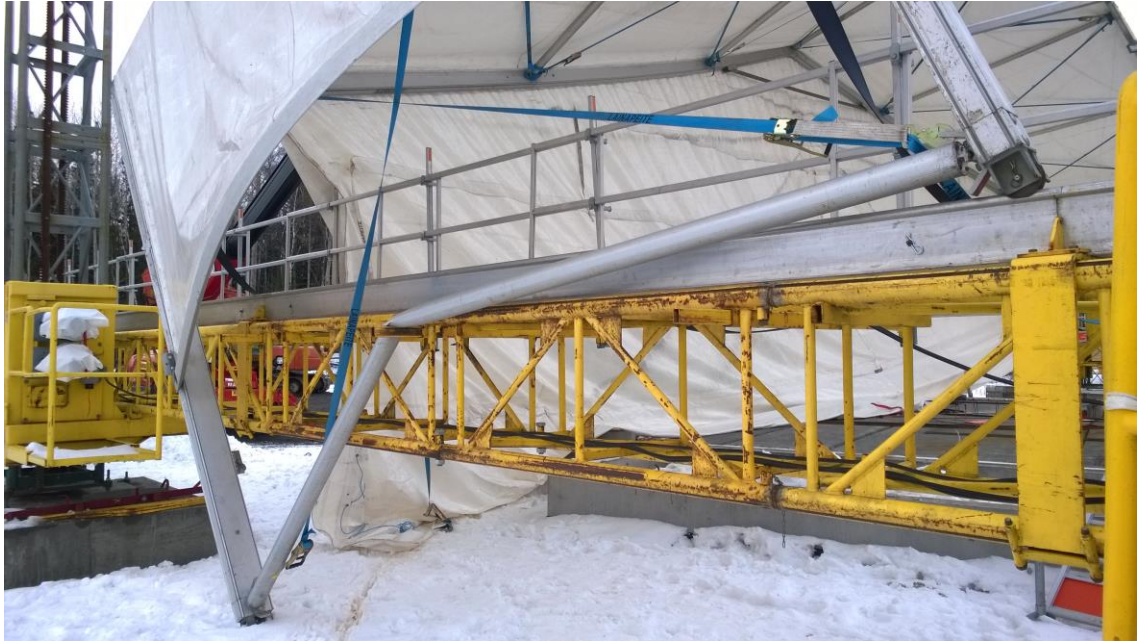
Figure 6. A derailing damaged a horizontal brace and caused a danger of the roof module falling down on its side.
