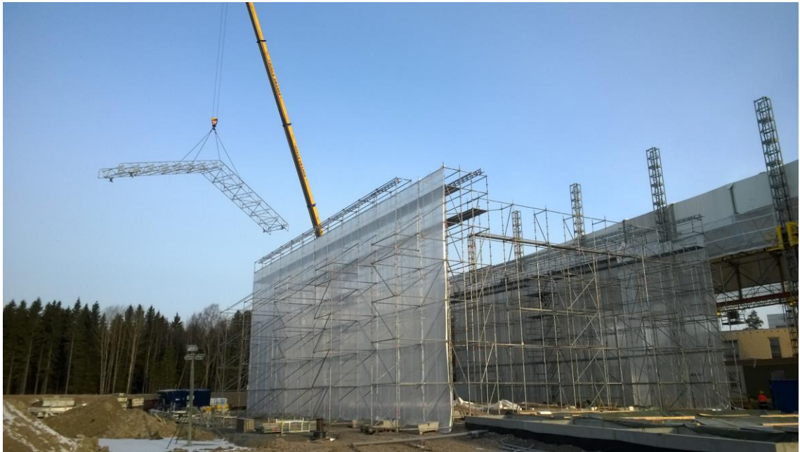
Figure 11. First Keder Roof module being lifted to its place after being assembled next to the cover system. The two separate rails for the separate roofs can be seen on top of the scaffolding.
