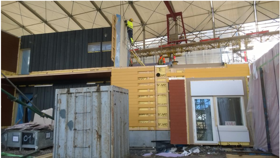
Figure 10. The bridge crane operator detaching the crane from a small external wall element after the element is temporarily supported.
