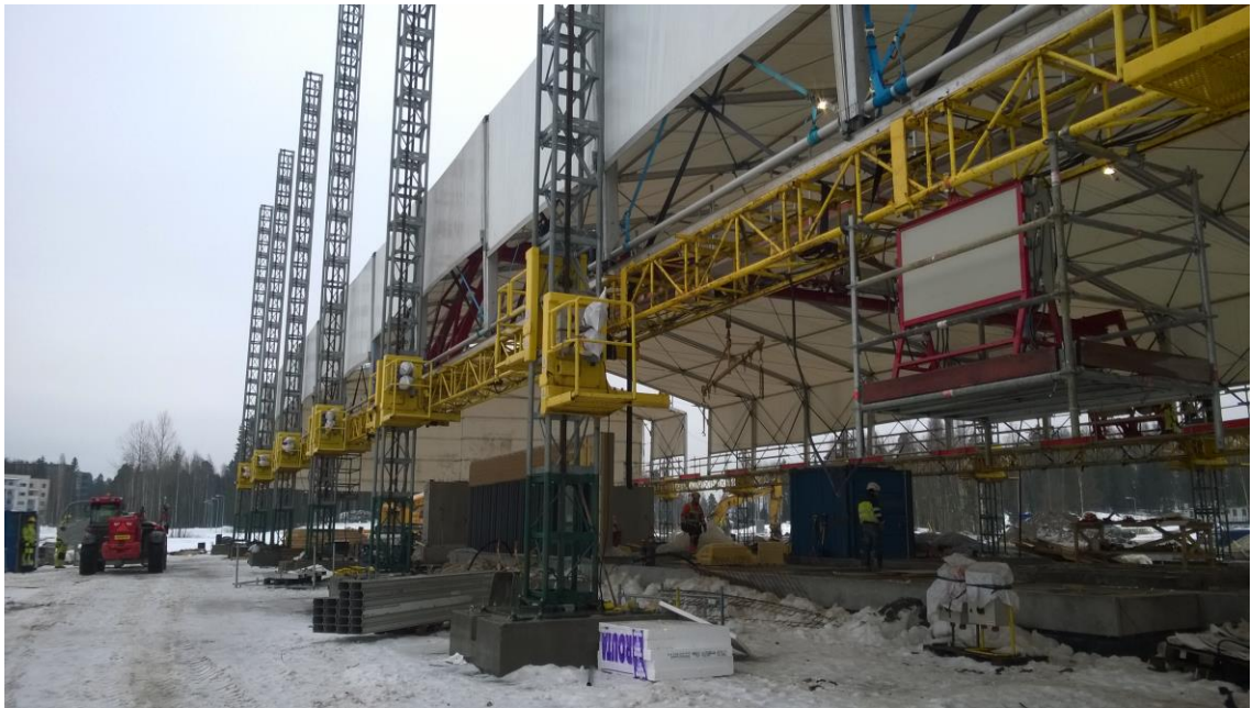
Figure 7. An electrical motor stuck lower compared to the other motors.
