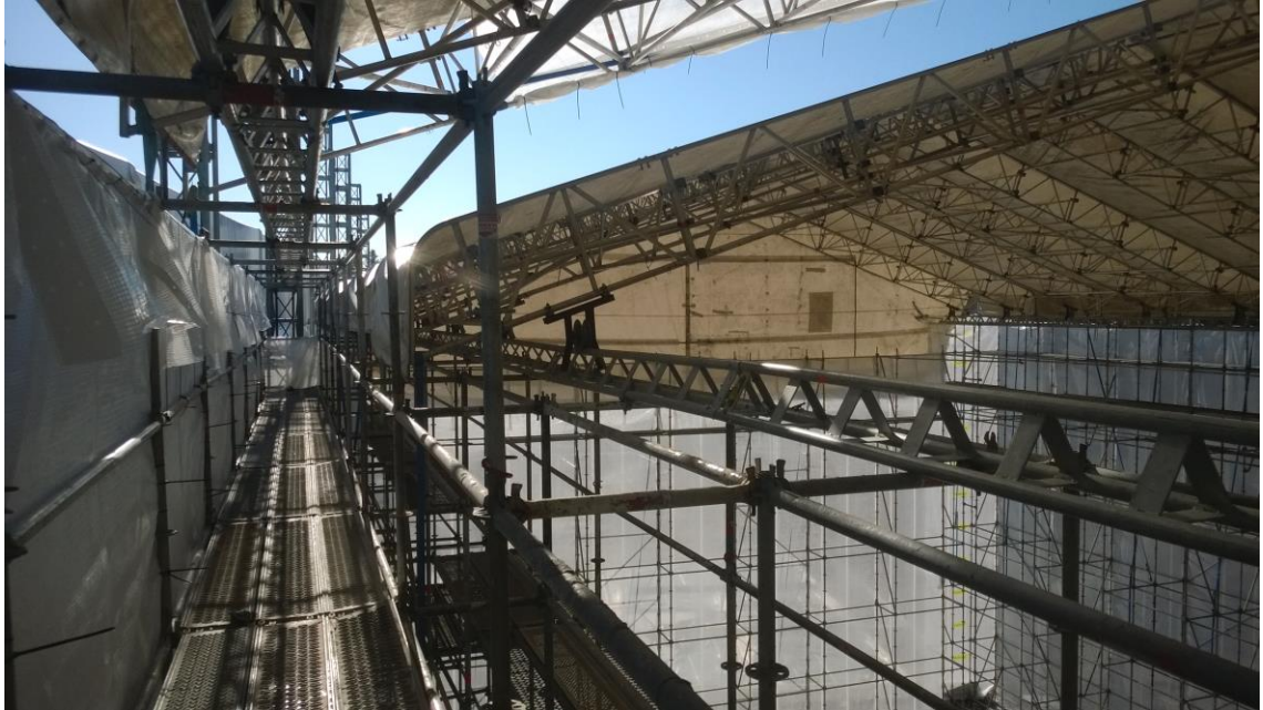
Figure 12. The two separate roofs on their own rails. The higher roof rests on the outer rails.
