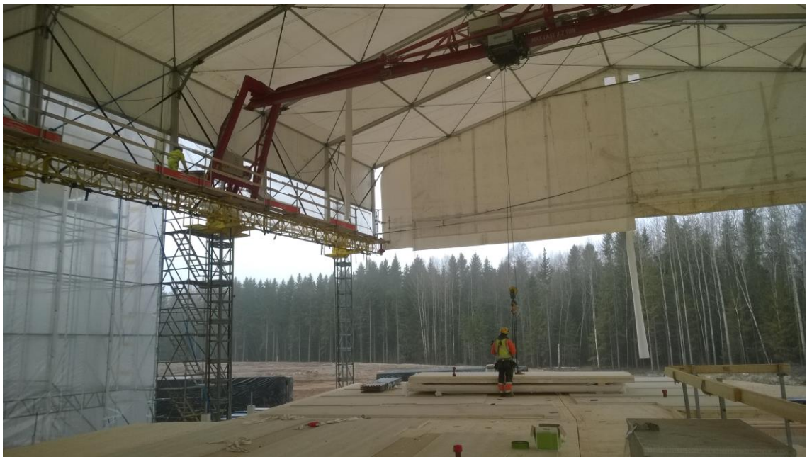
Figure 8. Operator of the bridge crane preparing to lift a balcony floor element. A worker of the company providing the weather cover systems up at the crane making sure the cable stays on right track.
