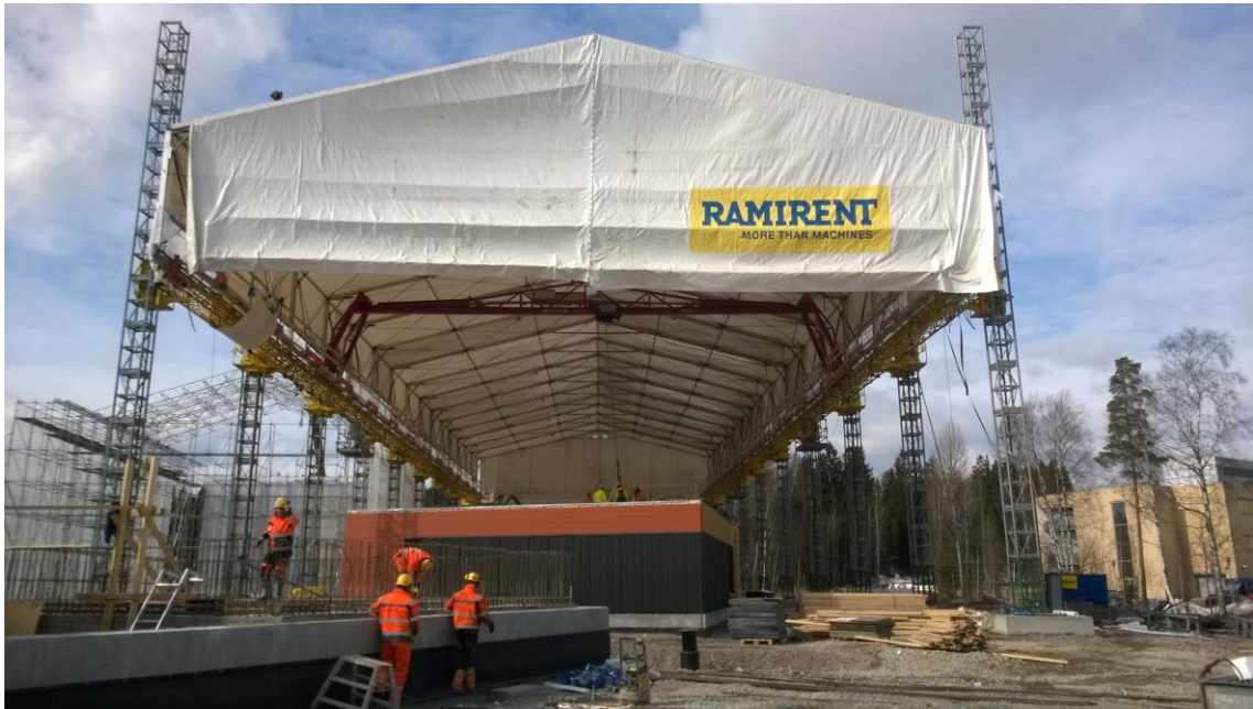
Figure 2. Gibson Tower in use. Wooden elements of the first floor are partially installed.
