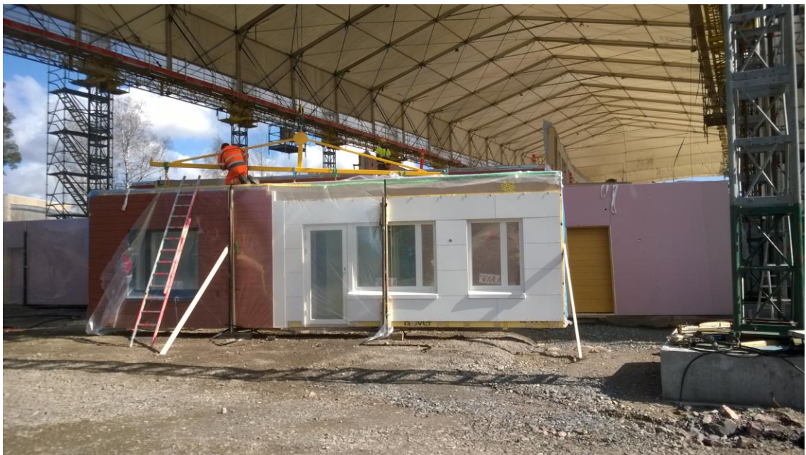
Figure 9. Wall elements moved underneath the cover system for lifting. An element is being prepared for moving to its place. The elements are temporarily supported.
