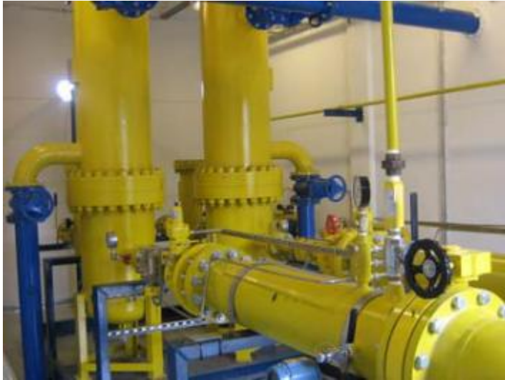
Figure 28. Gas pressure reduction unit. /63/
