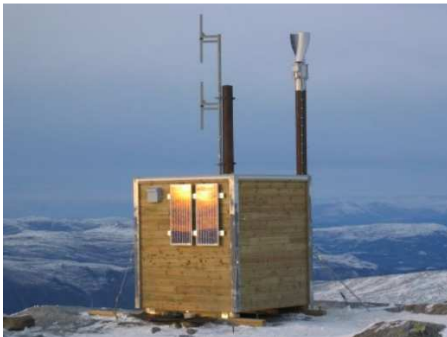
FIGURE 34 Windside WS-0,15B wind turbine producing power for a police repeat station in Norway (Oy Windside production Ltd, links Tuotteet.)
