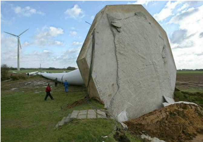
FIGURE 27 Catastrophic failure of a wind turbine foundation. (Miceli 2013.)
