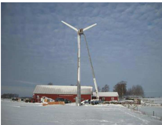
FIGURE 37 Windon 20kW installed in Wadstena, Sweden (Windon AB, links Vindkraft -> Bilder.)
