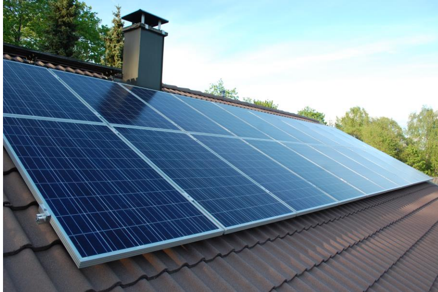
Figure 6. Solar panel array
