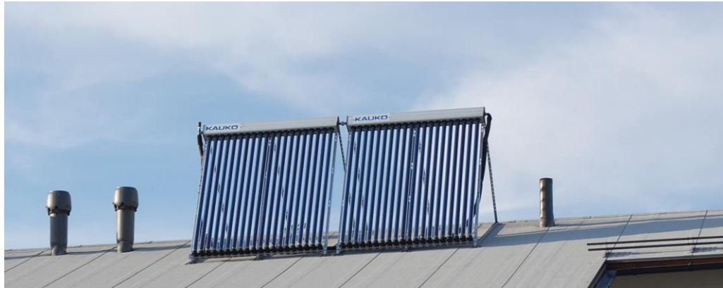
Figure 4. Solar collector with heat pipes
