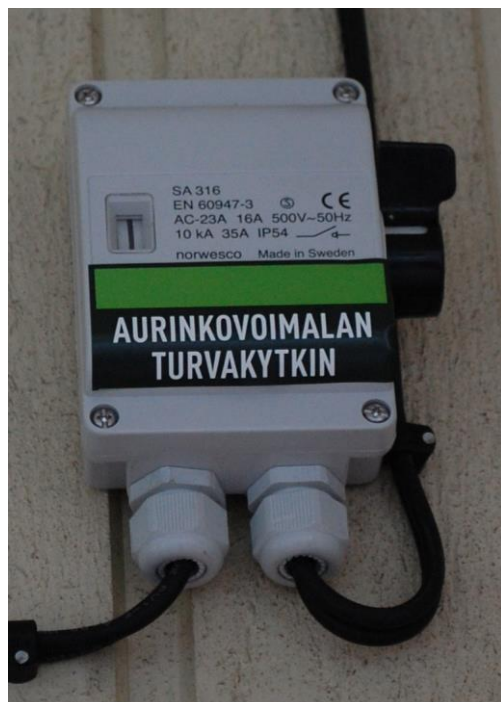
Figure 28. One type of safety switch situating outside the building
