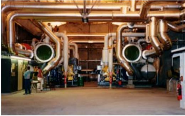
FIGURE 14. Sandvika Wastewater energy central in Oslo (Friotherm) /4, p.6/
