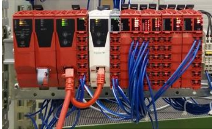
Figure 20: Example of connected TM5 safety logic system
