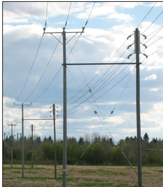
Figure 20. 1x20kV with 110kV cross-arm setup next to 20kV 2xPAS. /34/
