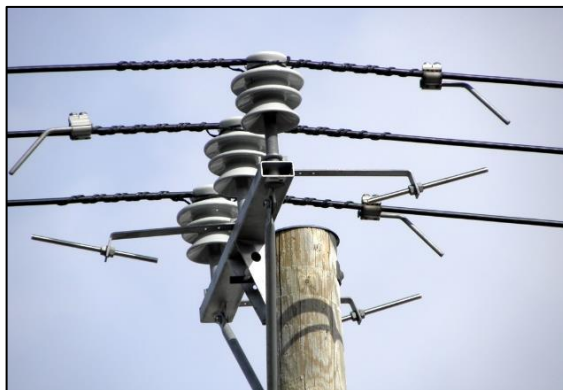
Figure 11. Power arc device installation. /15/
