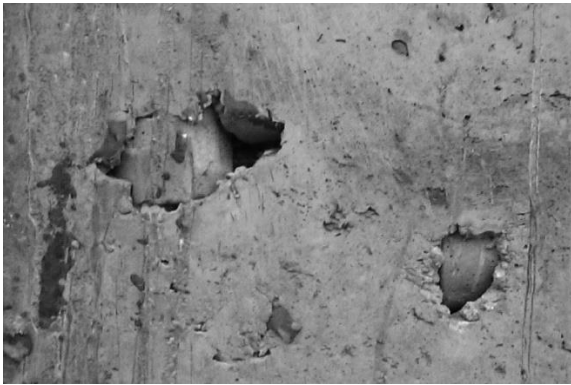
Inappropriate use of steel rod's fixation
