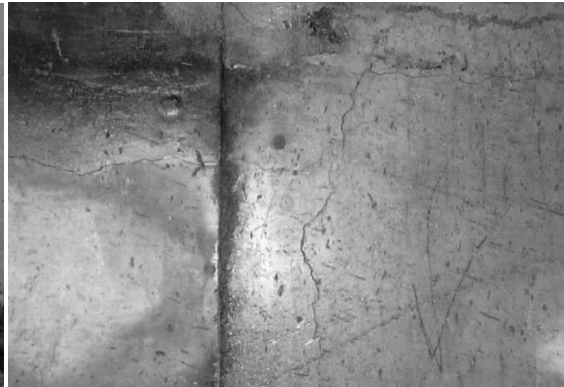
Cracks due to the shrinkage
