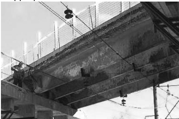
Concrete covered in mold
