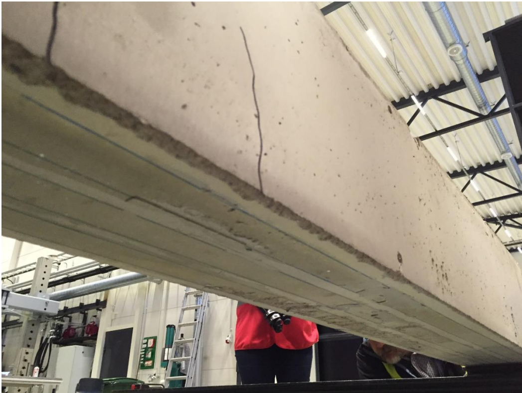
Reinforced beam 1 failure mode
