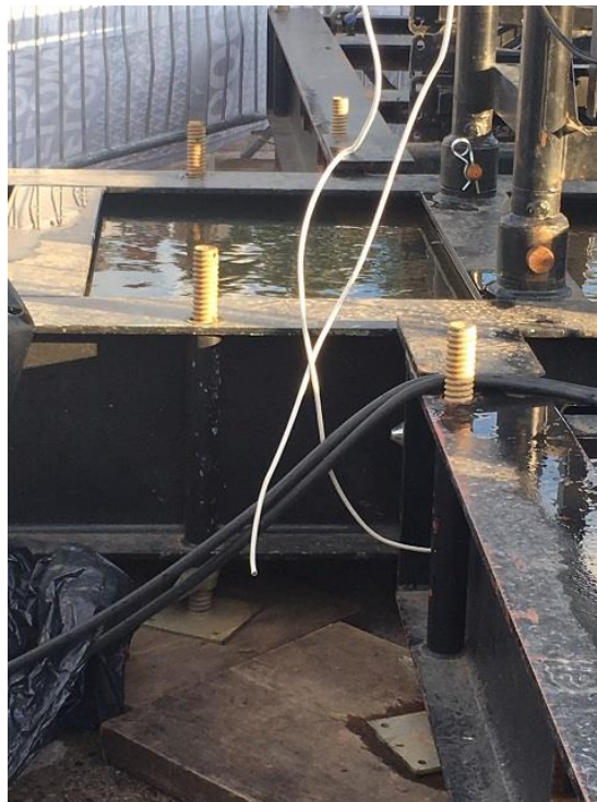
Figure 33. Cause of connection problems
