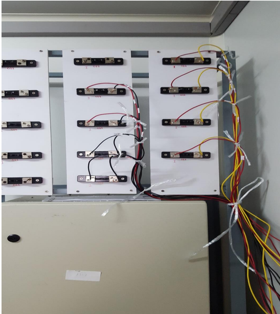
Figure 5. Rack for shunt resistors
