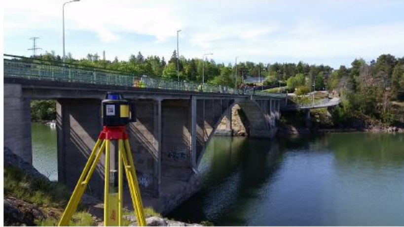
Figure 1. A rotary laser forming a reference level for a DMM sensor assembled in the middle span of the arched bridge.
