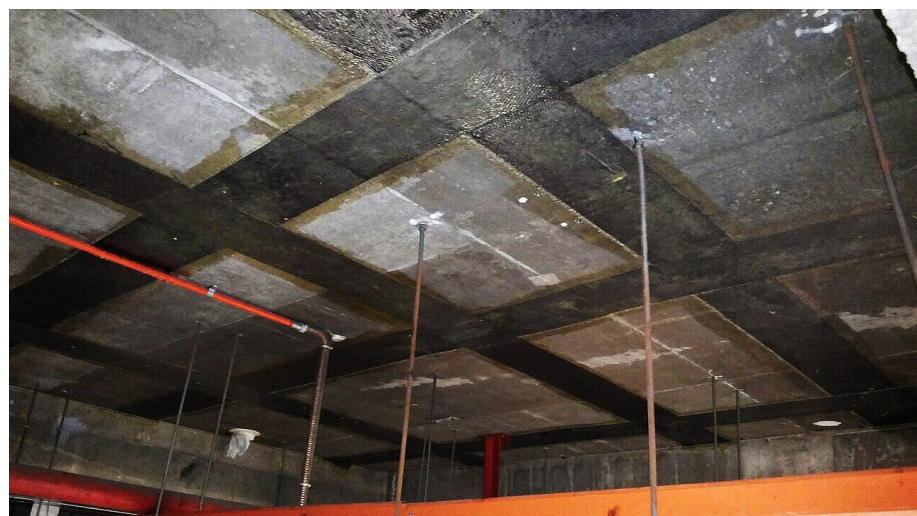
Figure 17. Example of Fibre Reinforced Polymers strengthening
