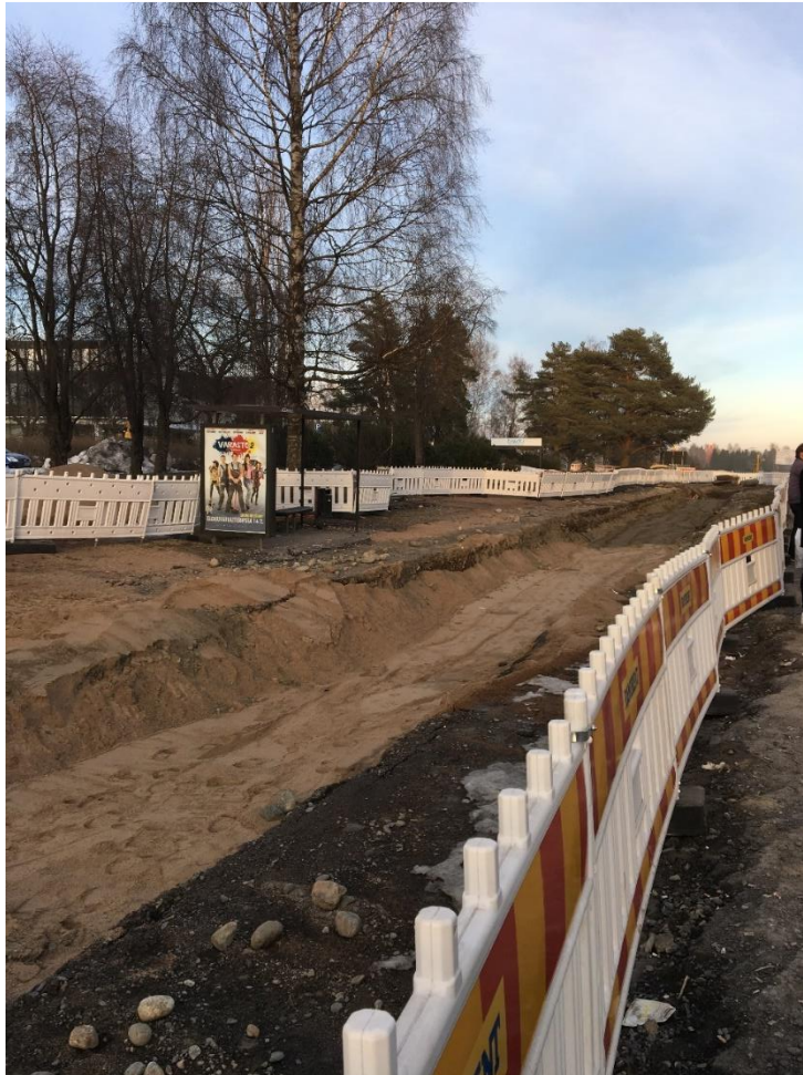
Image 5. Tram constructions on Sammonkatu. A bus stop is not in use and a large part of pedestrian and cycling roads are under construction. (Mannila, M. 12.4.2018)
