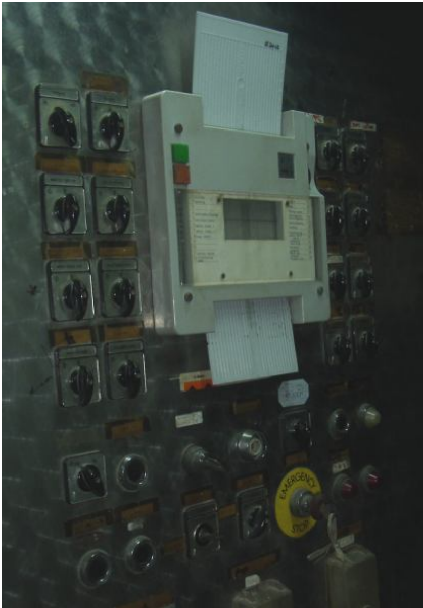
Figure 10. L.H. Lorch washing machine controls
