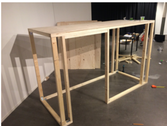
PICTURE 13. The wooden frame in progress. (With the ceiling board placed on top, but not attached yet.)
