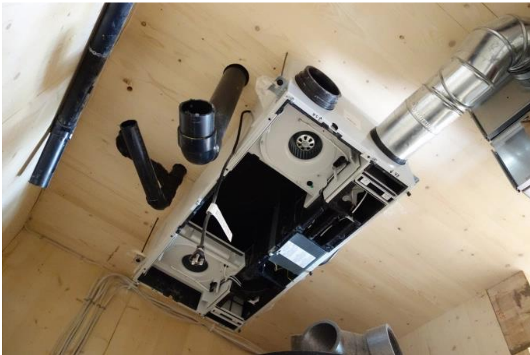
Figure 13. Ceiling mounted Zehnder ComfoAir 200 unit [37].
