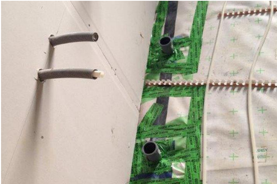
Figure 12. All pipes and tubes are properly air seal on the wall and floor [31].
