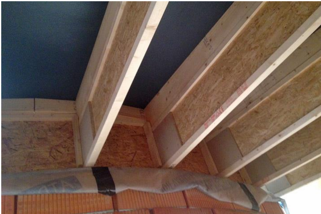
Figure 8. Overlap air seal over the top course of bricks to create continuity for ceiling air barrier [31].
