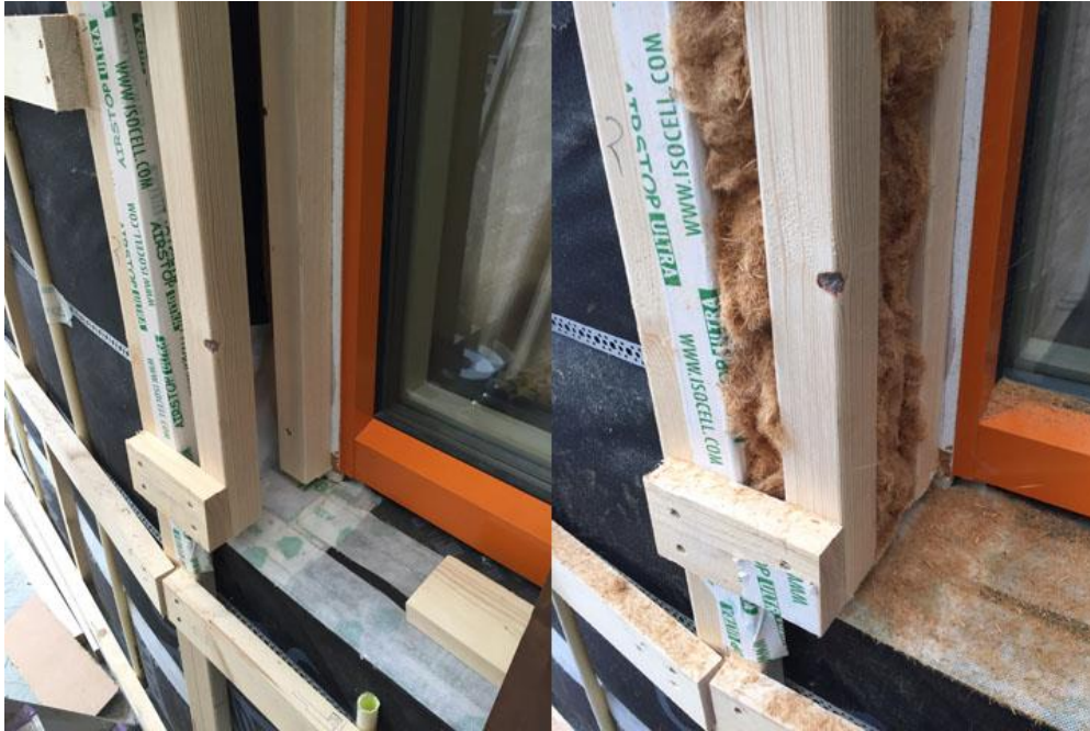
Figure 5. Window installation with proper air seal and insulation at exterior face of the frame [31].
