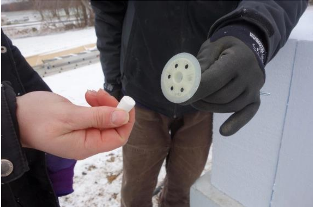
Figure 7. Plastic head covers and polystyrene plugs to prevent thermal bridges for EPS screws [36].
