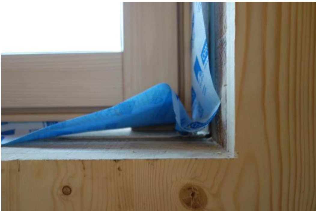
Figure 10. Gap at the window 12.5mm, which will be filled with a special expanding foam [43].
