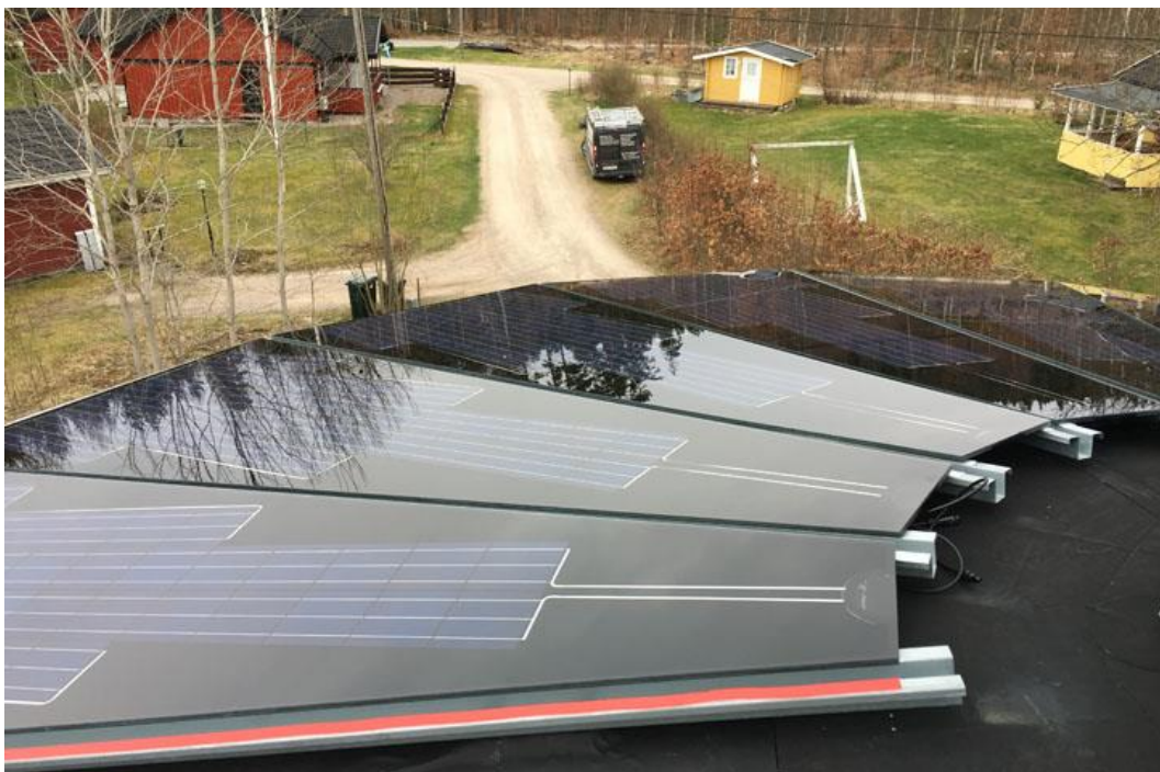
Figure 13. Solar panels on roof [31].
