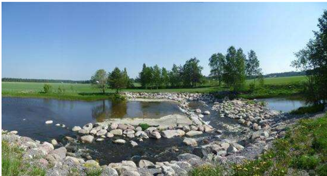
PICTURE 2. The bottom dam with fishway in The River Hirvihaara (Ympäristöhallinto 2014).
