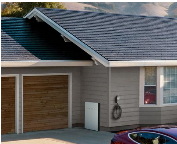
Figur 6. Teslas Powerwall-ackumulator installerad ute. /40/
