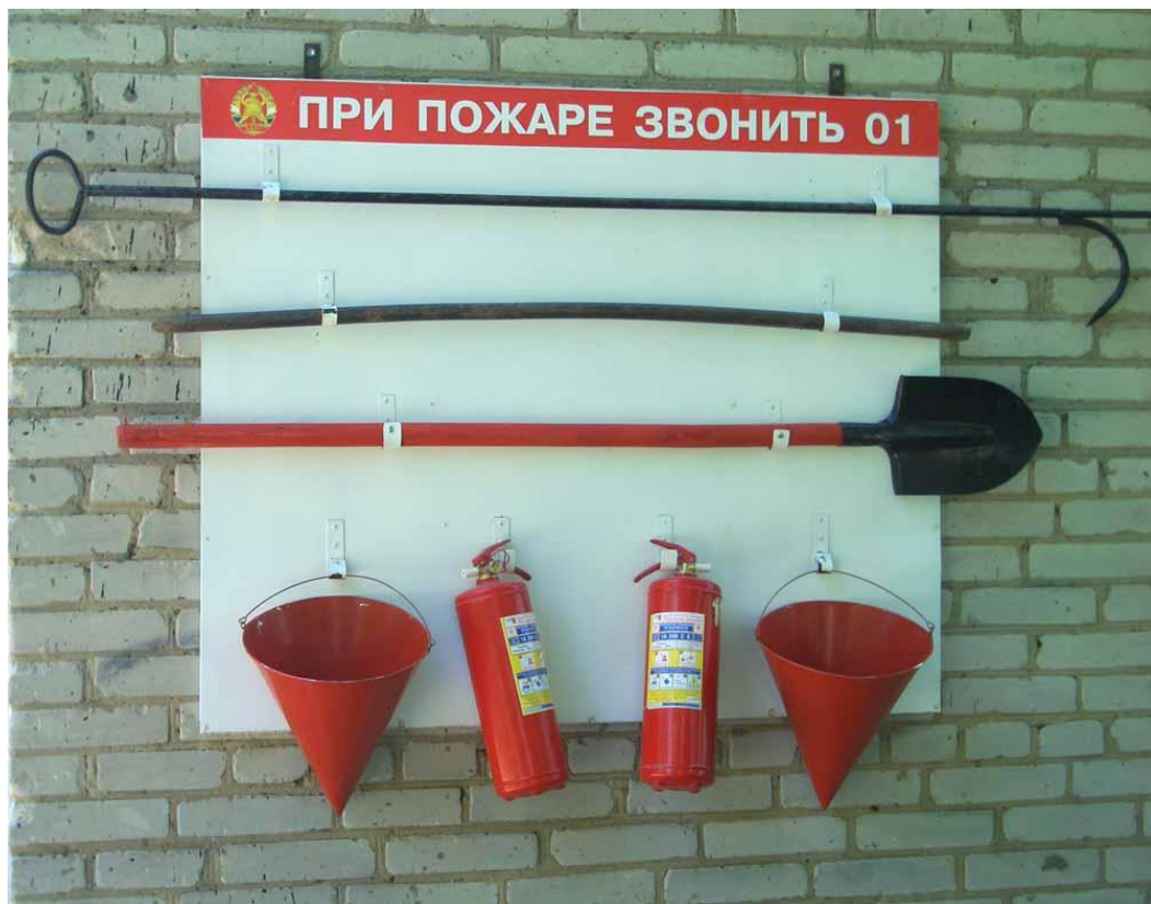
Figure 4.5 Fire shield on a building site ( http://www.movdpo.ru/stend22_06.html )
