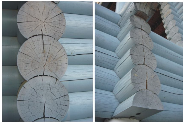
Figure 4.6 The cracks in the wooden elements on the opened terrace
