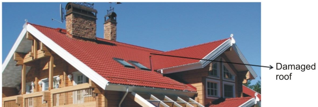
Figure 4.4 The place where the roof was damaged
