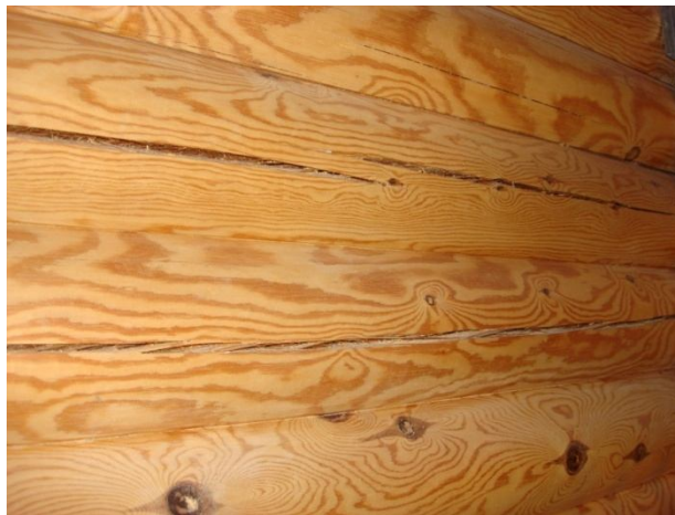
Figure 4.9 The cracks of the logs (inside the house)
