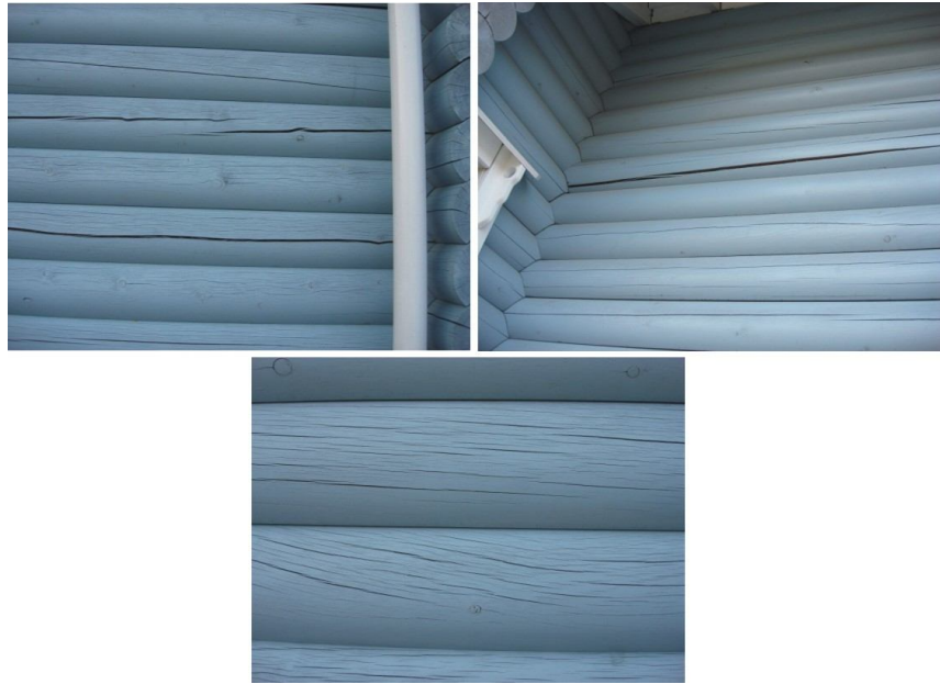
Figure 4.8 The cracks of the logs (outside the house)
