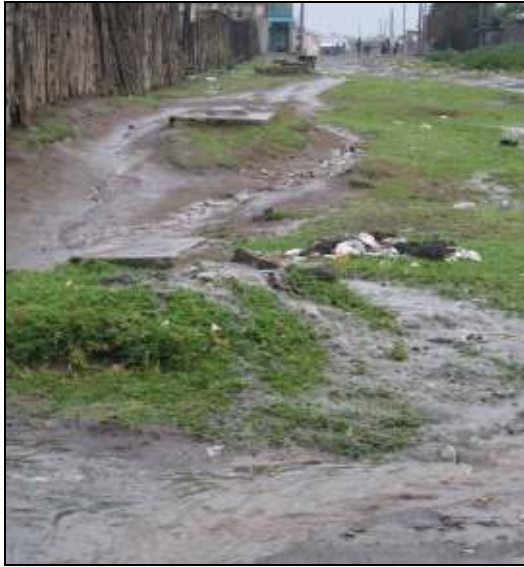
Picture 9: Many of the sewers are blocked and overflow during the heavy rain (Photo: Nurmi L. 2009)
