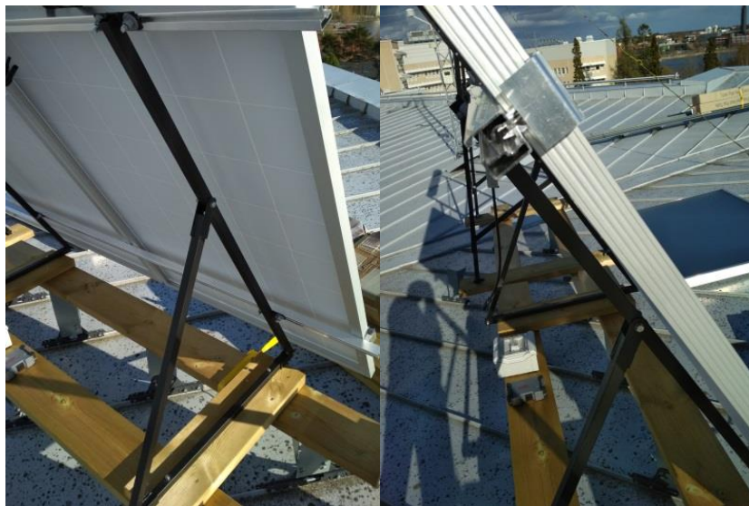
Figure 27. Metallic structure for the photovoltaic panels with an angle of 60^\circ .
