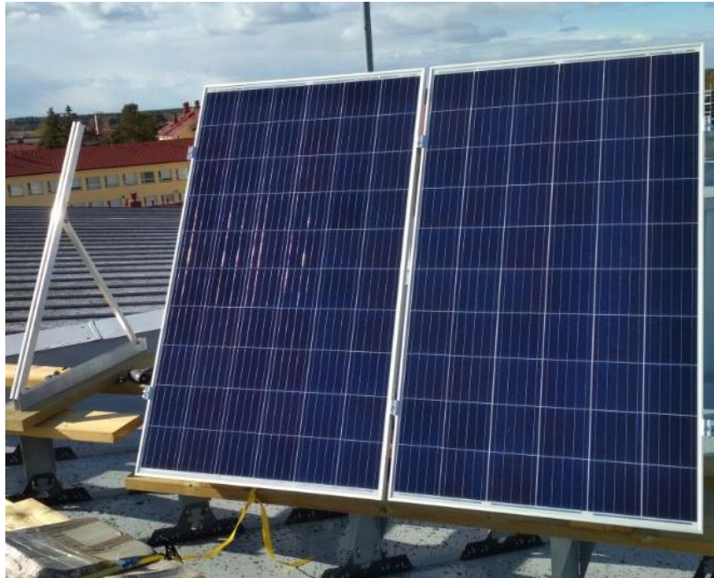
Figure 19. Photovoltaic panels Talesun TP660P-275 installed on the Novia roof.
