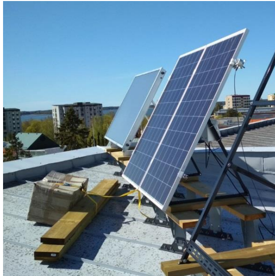
Figure 30. Solar thermal (in the back) and solar PV (in the front) panels on the roof of Novia.
