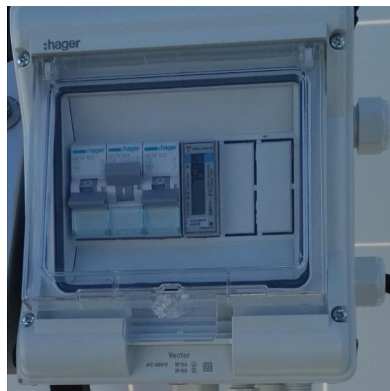
Figure 21. Energy meter Carlo Gavazzi Type EM111 (center of the picture) installed in a protection box.
