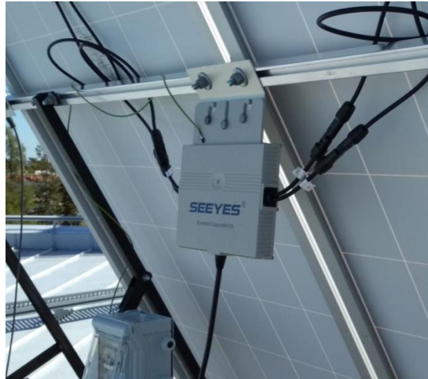
Figure 20. Installed ENVERTECH EVT500 Microinverter.
