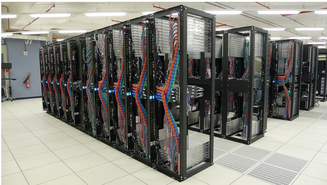
FIGURE 2. Server racks in a data center [5]
