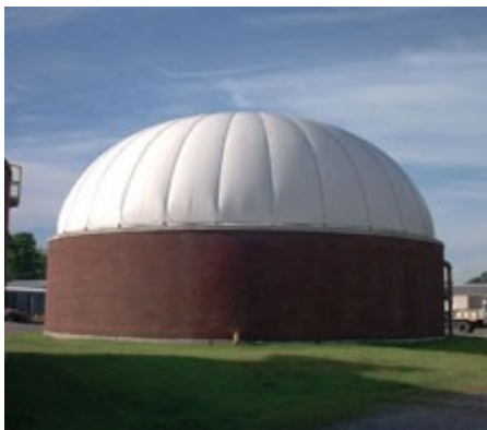
Figure 3: Internal biogas storage (Siemens Water Technologies 2011)
