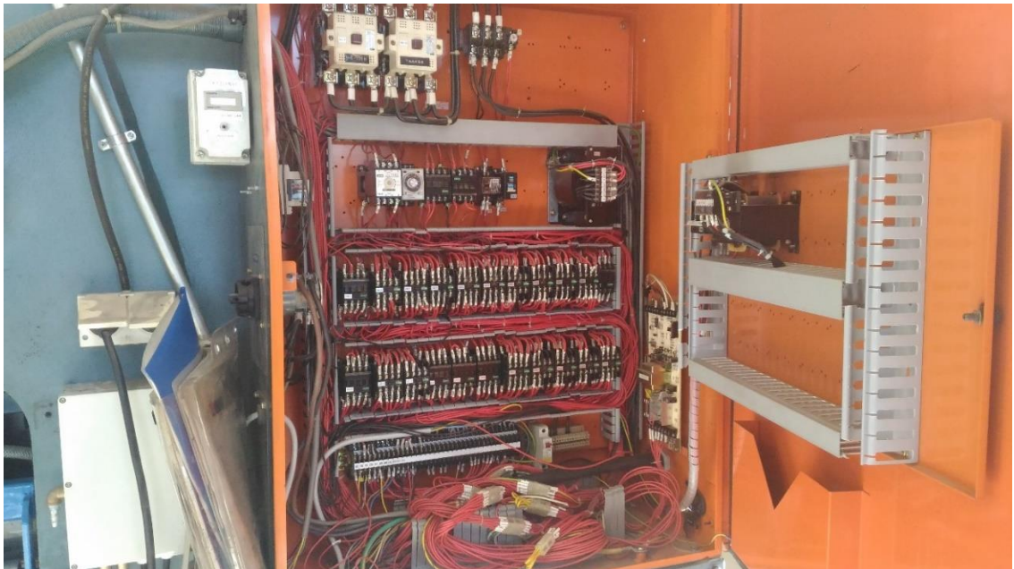
Picture 12. The old contactor control system within the electrical cabinet.
