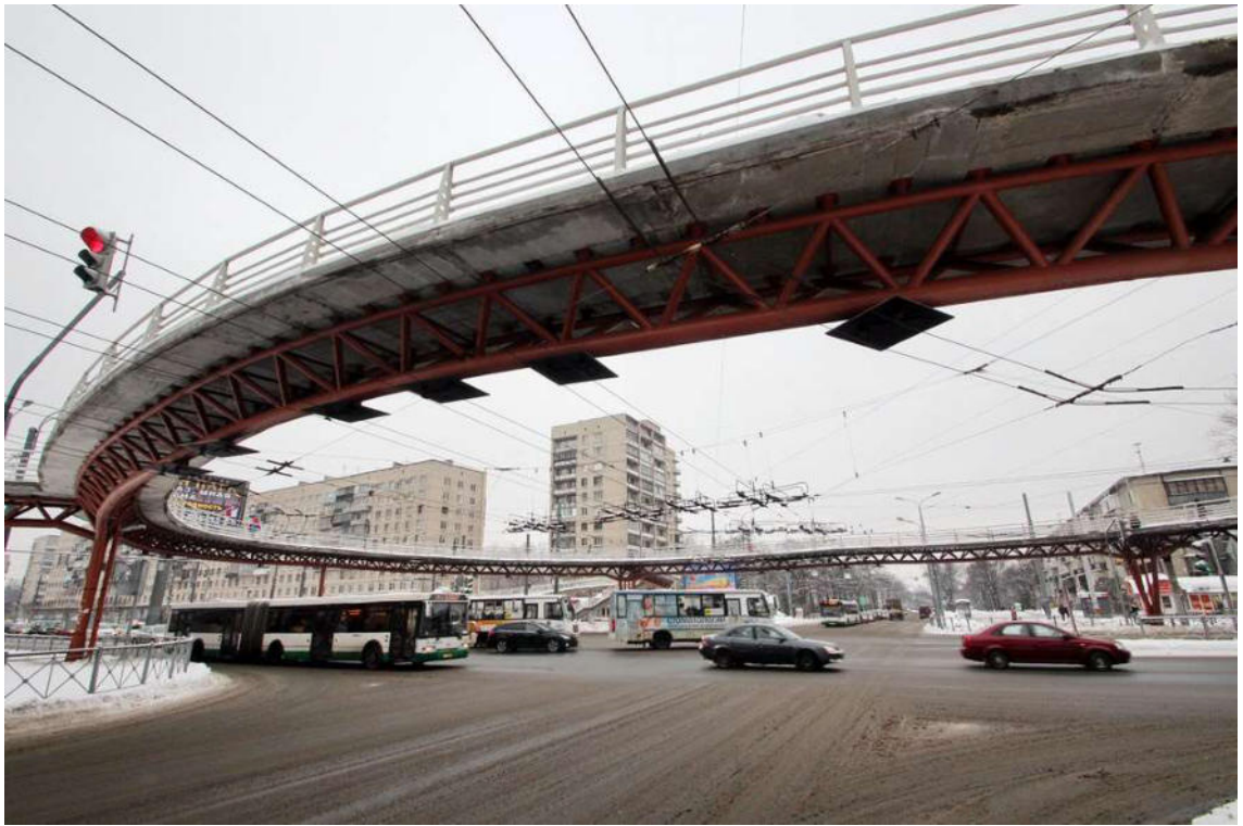
Figure 8.10 View on the circle overpass from the corner of the Budapeshtskaya street (image from kanoner.com)
