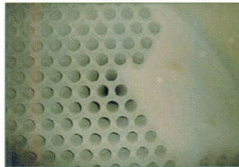
Fig. 2: Smoke tube boiler inside, after 7 days below 40% load. Limited soot deposits.
