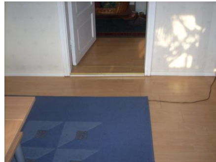
Alakerran lattia on painunut
