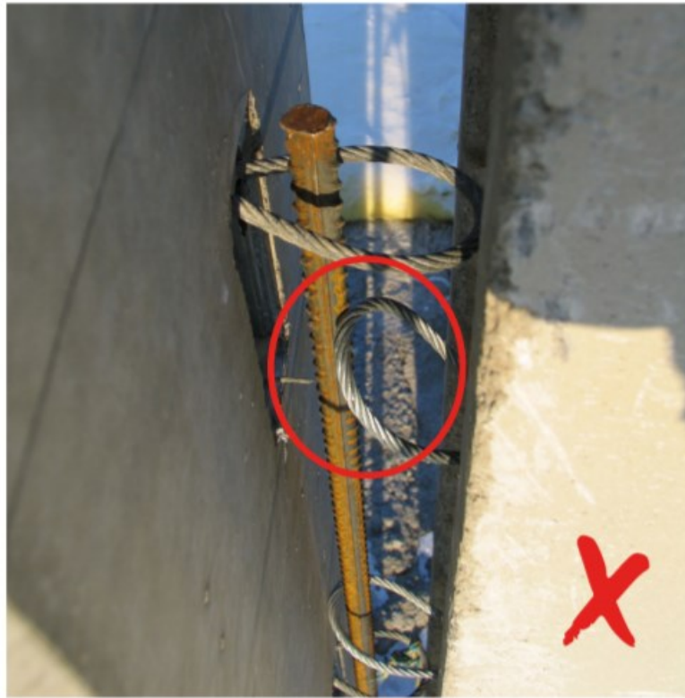
Figure 51 Incorrect installation of wire loops (Peikko, 2019, p. 26)
