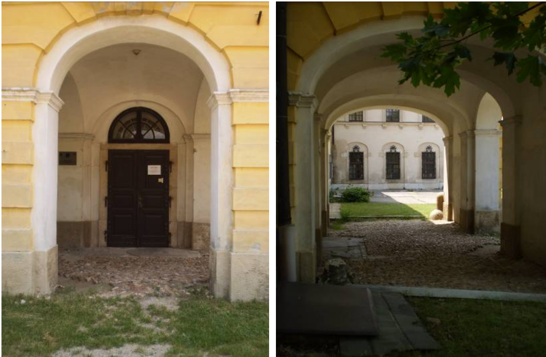
Figures 5& 6. Views by the main entrance, photos taken by Annika Pöyhtäri in June 2010.
