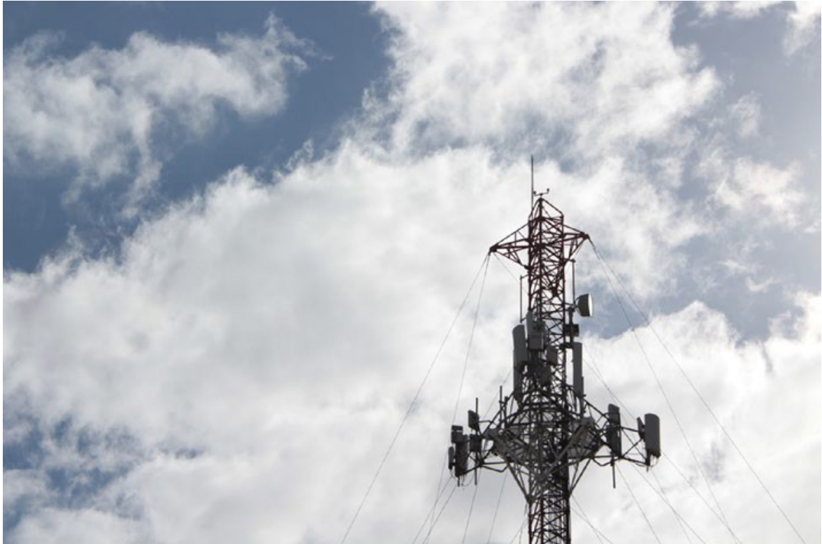
Figure 3. A cell tower [2].
