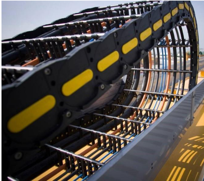
Figure 11 RTG trolley cable track (Rubber tired gantry cranes, 2012)
