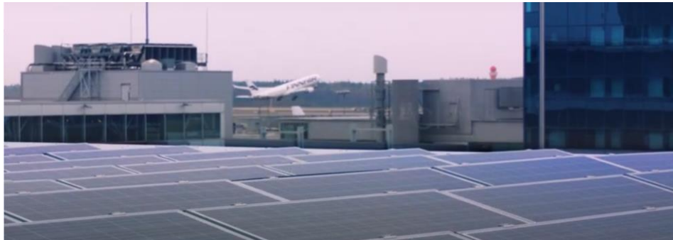
Figure 15. Finnavia's solar power plant on the roof of Terminal 2/ Finnavia [52].
