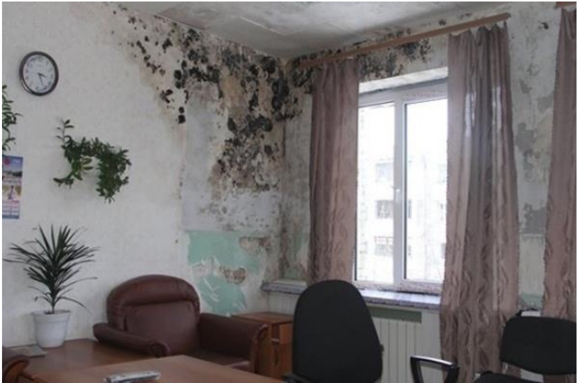
Figure 6. Mold problems in Hrustsevka
