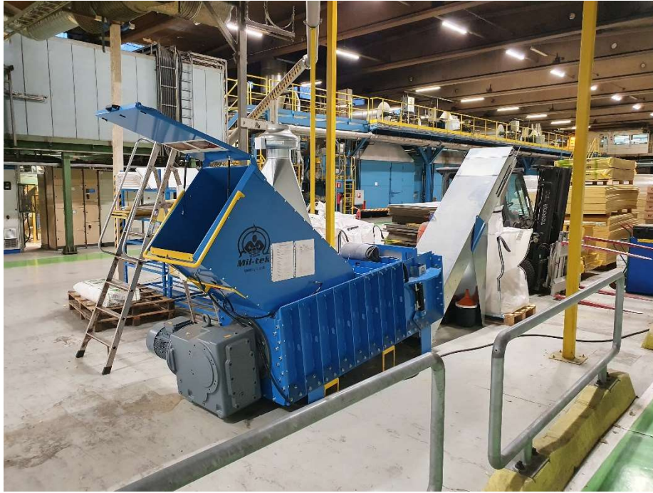
Figure 7 Mil-Tek IC60 situated on the ISOVER factory floor (Kohvakka, 2020)
