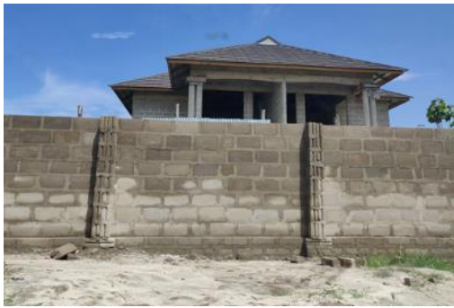
PICTURE 19. A house made out of sandcrete blocks under construction in Bagamoyo, Tanzania. (Mjema 2018)
