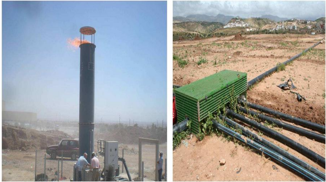
Figure 21: Flaring and collection systems in Bekarane site confirming biogas potential
