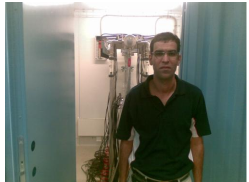
Inside biogas plant
