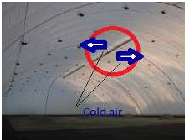
Figure 7. Distribution the cold air by special DUOL's pipe /10/
