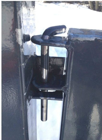
Picture 10. Gate locking mechanism. Merisatamanranta, Helsinki.
