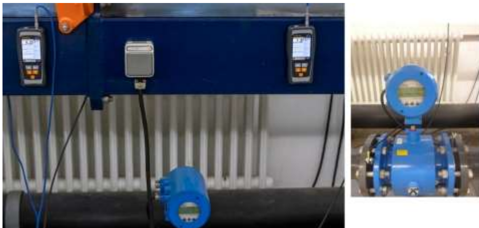
Figure 27. Set up of Magnetic Flow Meter and Propeller Flow Meter (HS Mainz, 2020)
