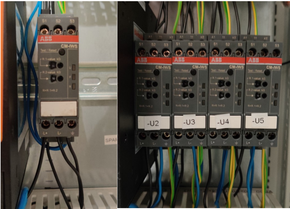
Figure 25. ABB CM-IWS.1S IMDs installed in the UNIC power supply cabinet.
