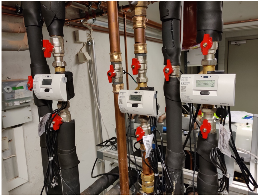
Figure 1. Water circuit pipes of the adsorption chiller system and the energy meters connected to them.
