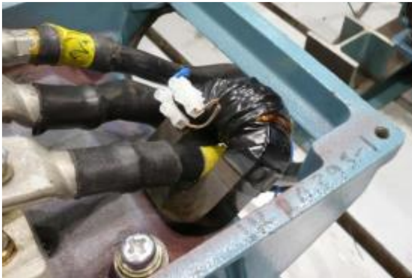
Figure 6. Current transformer installed around the motor phase conductor. /7/
