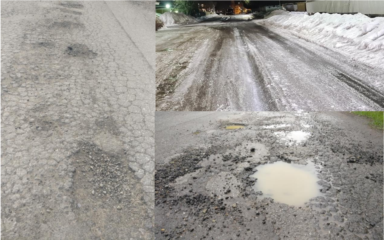
FIGURE 1. The outcome of using the traditional method of de-icing asphalt pavement
