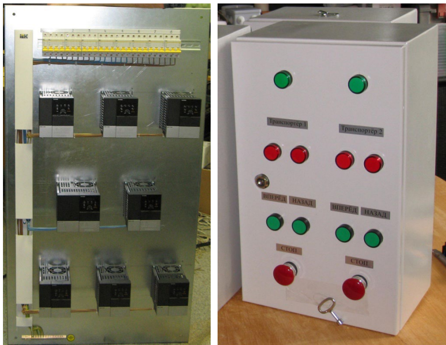
FIGURE 6. Frequency Converter Control Cabinet
