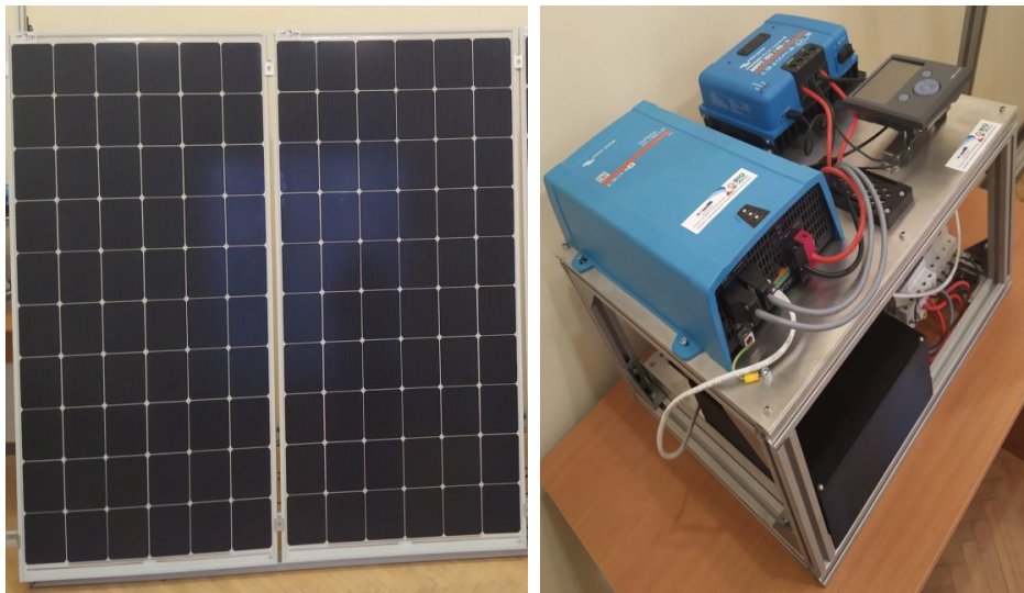
FIGURE 8. Photovoltaic Power Station
