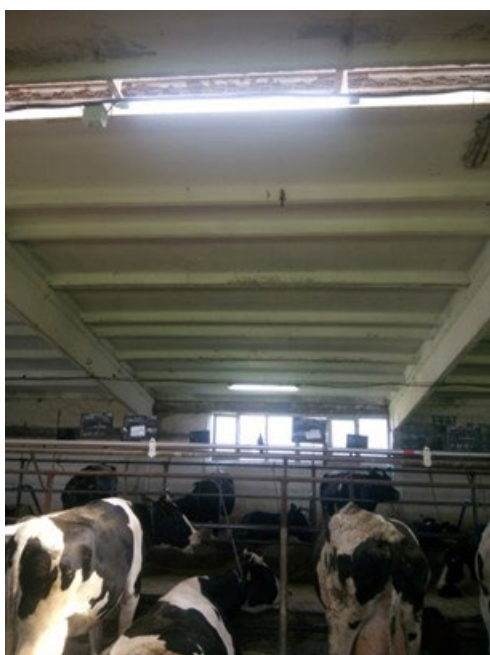
FIGURE 5. Lighting of Cattle Barn with LED Lamps
